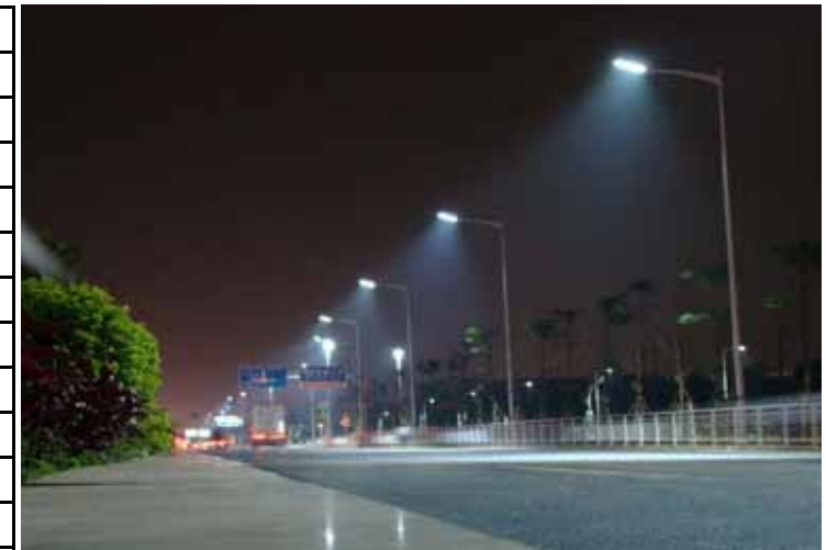
The 1st LED streetlight project in Shenzhen, Tangming Rd.
